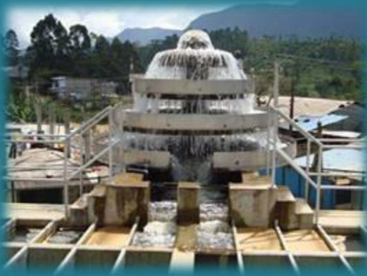
WATER TREATMENT PLANT AT MASKELIYA, MASKELIYA WSS
