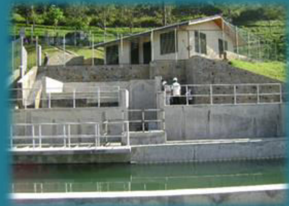
WATER TREATMENT PLANT AT HEWAHETA, RIKILLAGASKADA WSS
