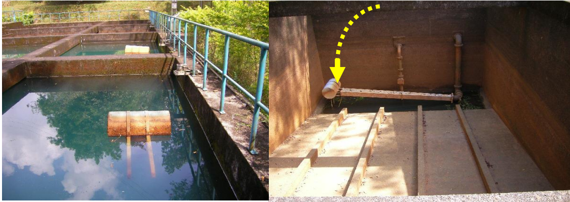
Moving inlet pipe with pontoon with hinged bend (Kalatuwawa WTP: 1954)
