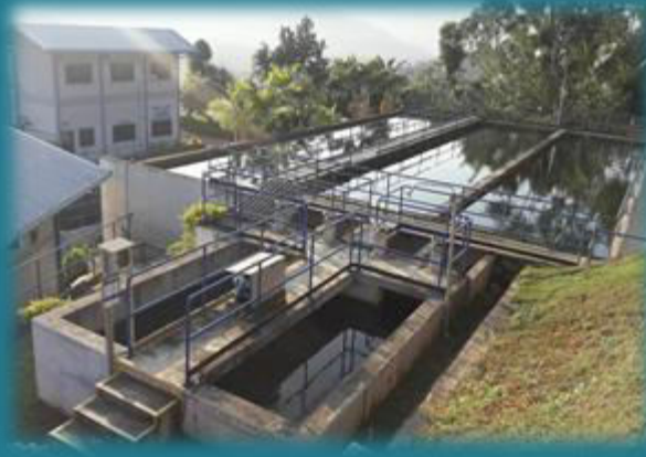
WATER TREATMENT PLANT AT PARADEKA PARADEKA WSS
